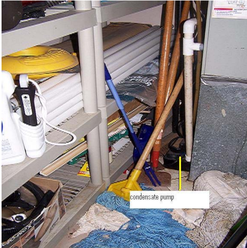
Photo 1: HVAC Condensate Pump
