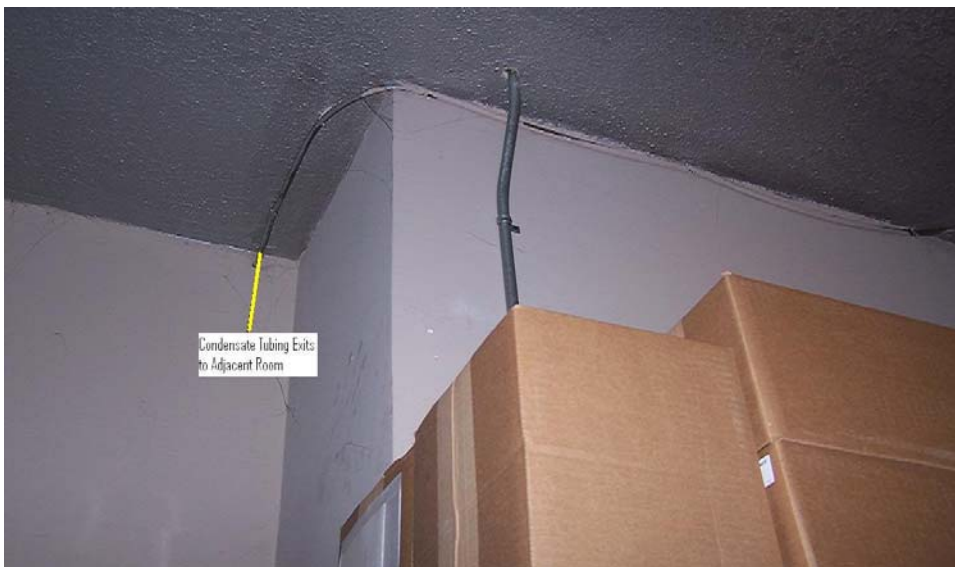
Photo 3: Condensate Tubing Along the Ceiling
