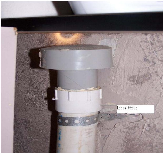
Photo 5: Loose Fitting For Air Admittance Valve
